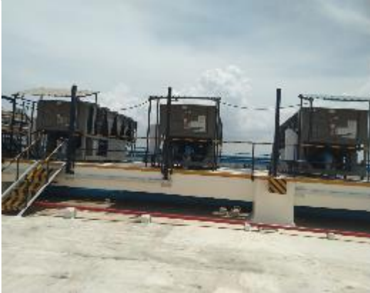
Switching off Ideal Chiller
